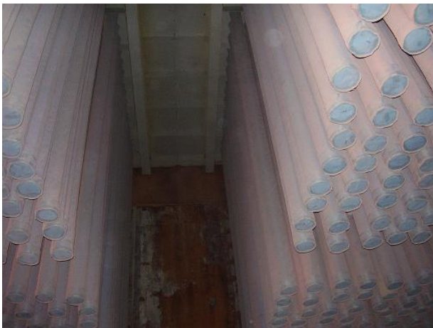
Figura 7 – Filtro com as mangas instaladas
