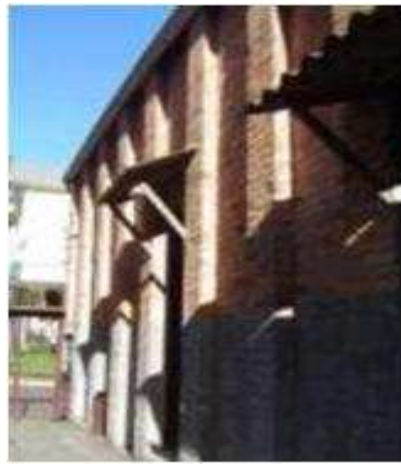
Figure 7 Galópolis Village houses - Source: Fernanda Poloni personal archive / Architecture and Urbanism Course. UCS. 2008
