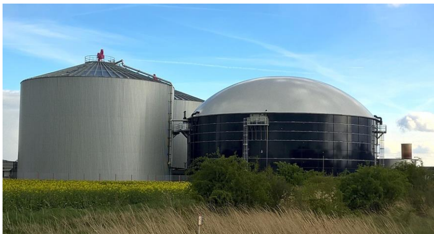
Figura 2 - Biodigestor Continuous Stirred Tank Reactor – CSTR
