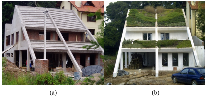
Figures 3.16 (a) and (b): Roof slab with barriers integrated, in a green roof in Nova Petrópolis, Brazil (The author, 2005)
