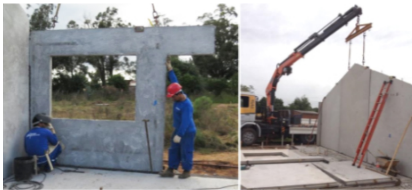
Figure 2.10: External walls of the constructive system, being assembled in the city of Candiota, Brazil (ACPO, 2014)
