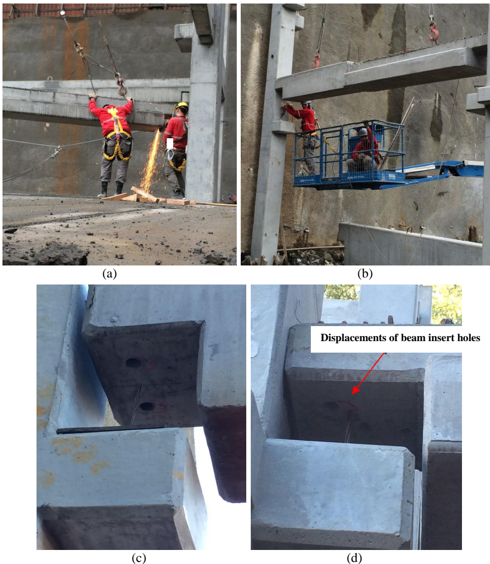
Figure 8 - Strategies adopted to cope with design and quality failures: (a) sanding one face of the beam to fit it; (b) installing a missing insert pin; (c) and (d) displacement of beam insert holes in relation to column insert pin
