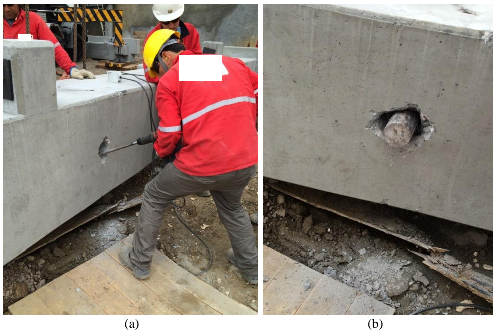
Figure 10 - Repairing a column: (a) assembler enlarging the column hole; (b) lifting pin placed in the adapted hole
