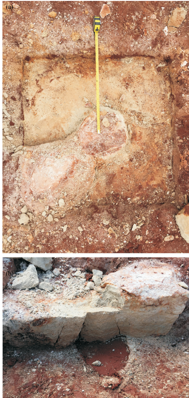
Figure 8. Photos of (a) the top view and (b) vertical cut in the middle of the 900-mm square and 300-mm thick Portland cement improved sand layer (coded L r 900H r 300 - SF) to check failure mechanism below the steel plate vertically loaded.
