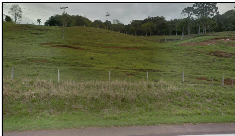
Figura 7-26 – Talude coluvionar na BR-386 (Google Earth)
